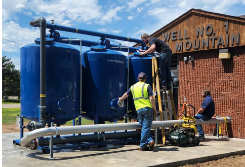
Photo of WaterSurplus PFAS removal system at Rib Mountain, Wisconsin
